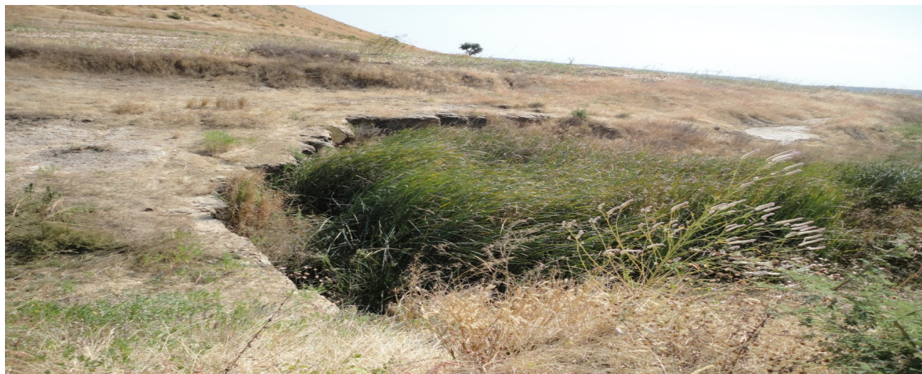
Plate-5 Shows fault plain along the proposed spillway area
