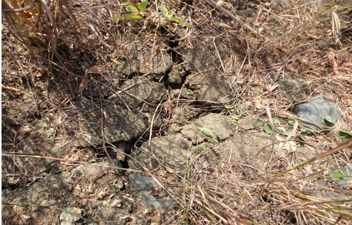
Plate-3 Shows Desiccated cracks within the reservoir area
