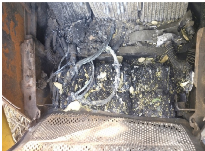
Figure-8: A view of burnt battery.
